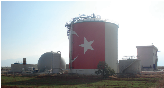
Konya Şeker Seydibey Solid Waste Treatment Plant 4.900 m 3 Anaerobic digester (100 ton/day organic waste; 1.700 kW heat energy), 2010
